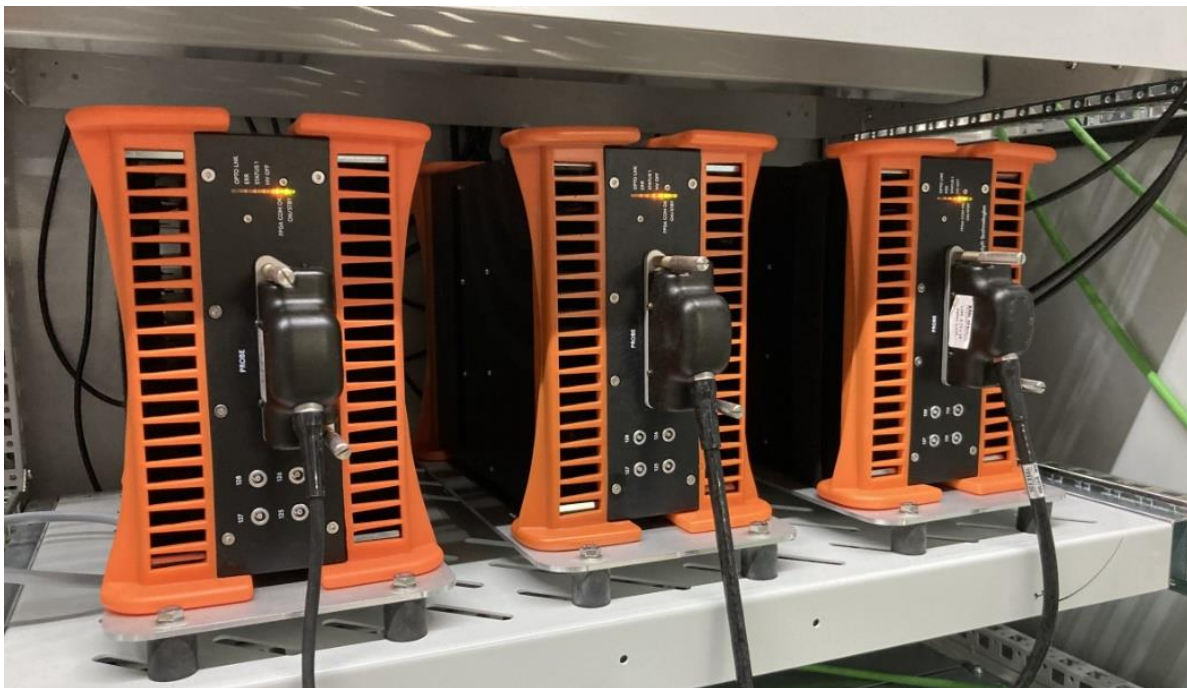
Fig. 9 ECHOGRAPH-PAUT electronic modules installed in a cabinet
